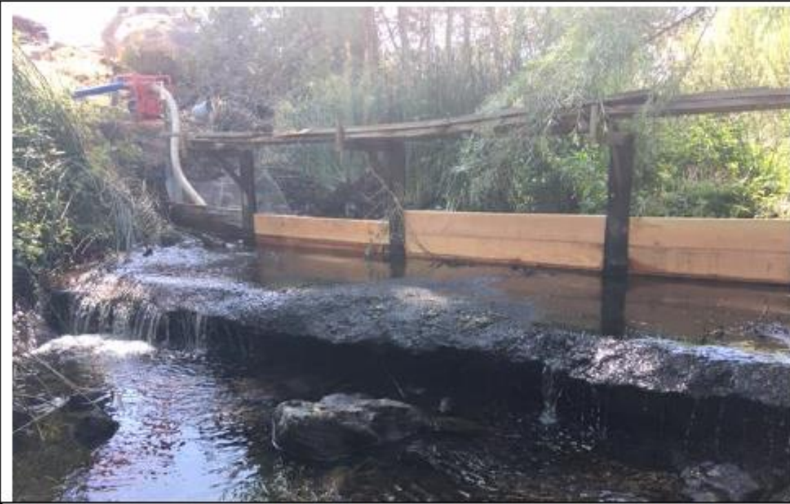
Photo Point 2- Pre project condition just downstream of the concrete sill and barrier looking south
