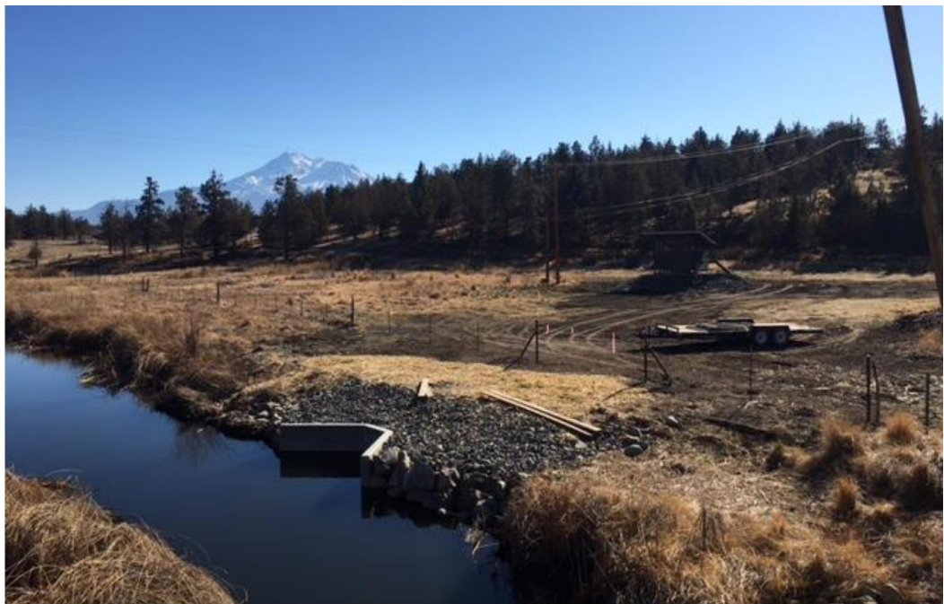
Fish Screen completed. Fencing and testing of the system to complete the phase.
