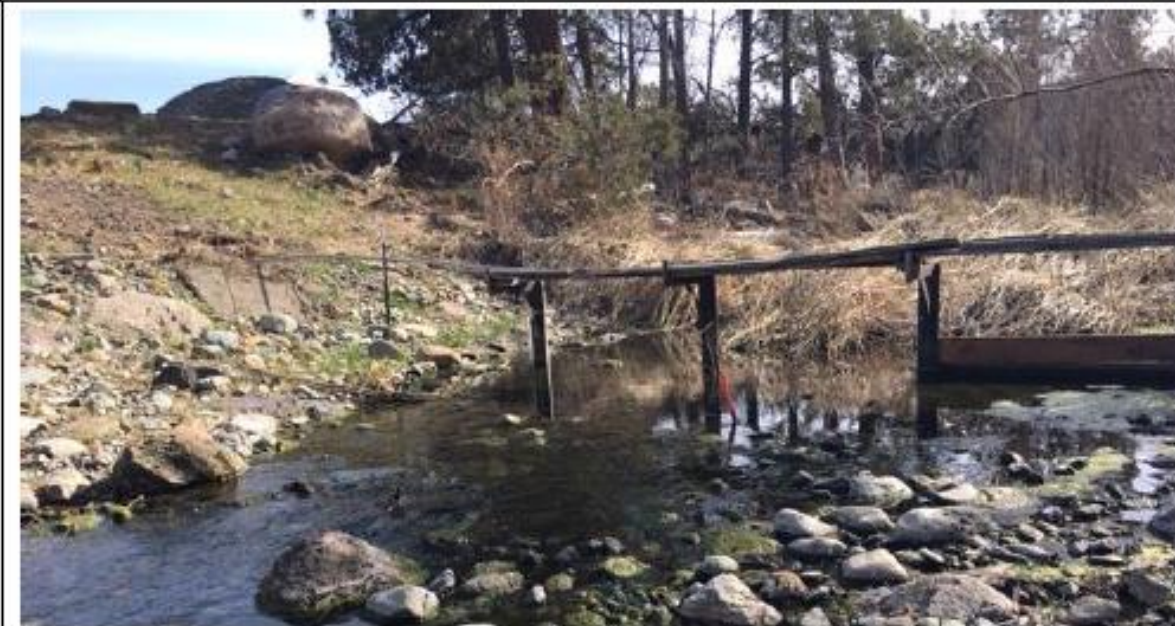
Photo Point 2- Post project conditions just downstream of concrete sill. Roughened channel backwaters the structure.
